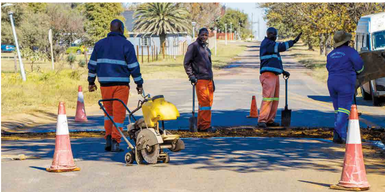
Roads Department employees in Hendrina busy erecting speed humps in Kort and Snyman Streets.
